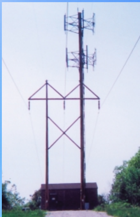
95' 138kV H-frame Transmission Structure with Two Antenna Arrays
