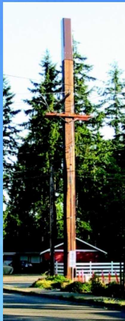
45' Distribution Structure with Concealed Antennas
