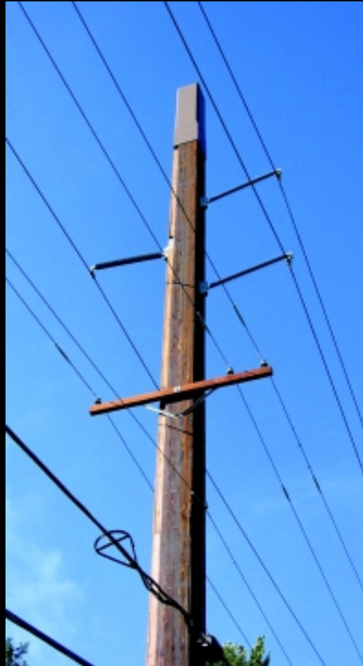
69' 115kV Transmission Structure with Distribution Underbuild, Cable TV Attachment and Concealed Antennas
