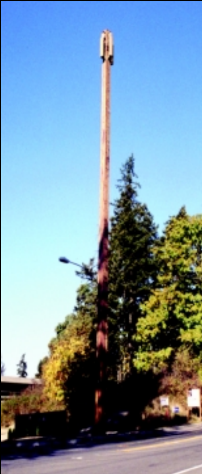
81' Distribution Structure with Street Light and Flush-mounted Antennas
