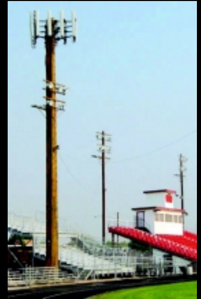
Field Lighting Structure with Single Antenna Array
