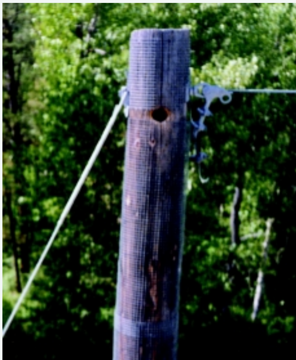
Woodpecker Damaged Round Wood Pole
