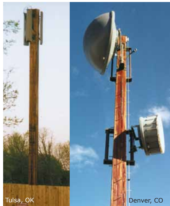
■ MONO POLE AND MICROWAVE TOWER
