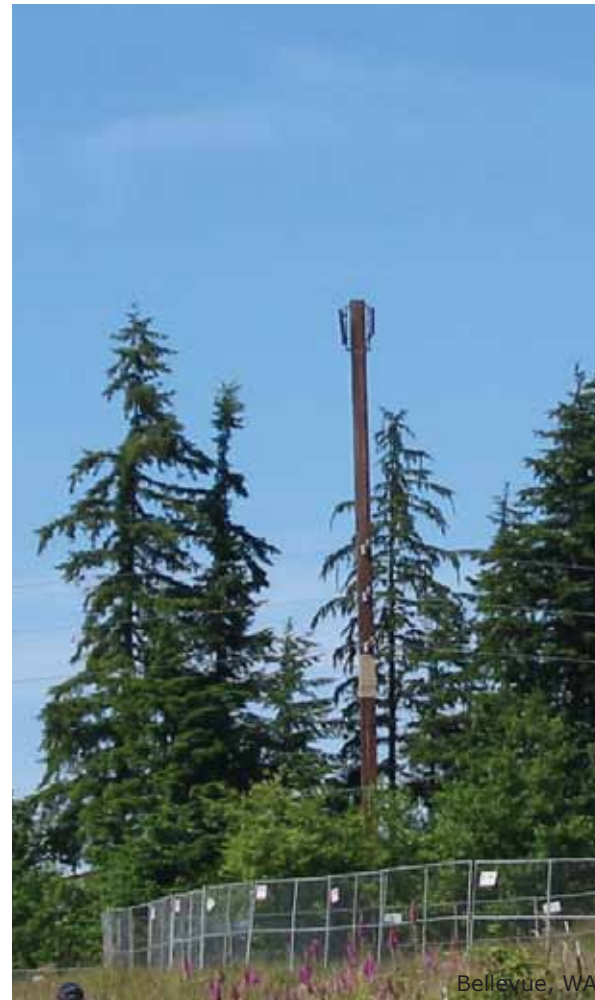
■ JOINT USE TOWER
