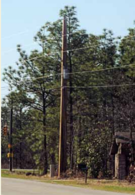
Laminated poles are much more aesthetically pleasing than steel or concrete poles.
