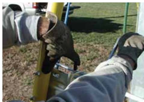
Lock winch pole winch in the raise position.
