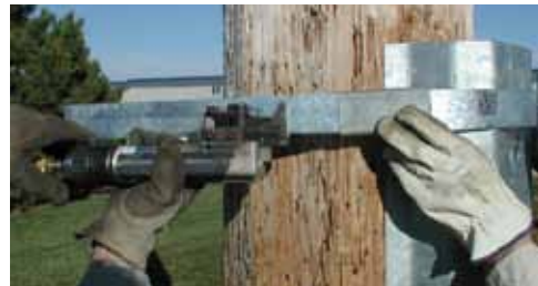
12 Tension the Banding using either an Air or Manual Tensioner.† Hit Banding with hammer to help tensioning.
