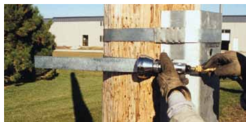
14 Cut excess Banding off next to Seal using Air Cutter or by bending back & forth with Tensioner still attached.†
