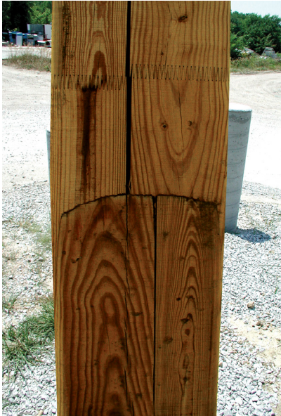
Photo A – Typical unglued edge joint on cut side of pole showing slight checking through thin area of next layup.
