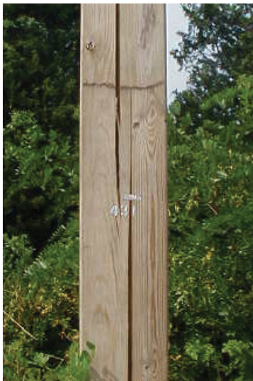
Photo C – Typical unglued edge joint on cut side of pole showing checking through thin area of next layup. Wood treated with CCA is more susceptible to deep checking than wood treated with Penta & Oil.
